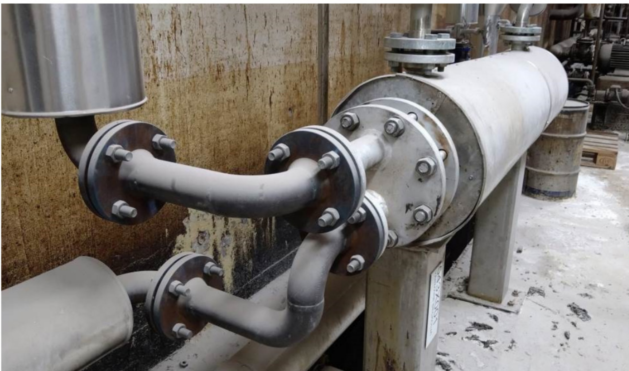
3. Shell and tube heat exchanger used for preheating tall oil pitch (shell side) in the Gruvön, Sweden, mill. Low pressure steam is used as the heating medium (tube side).
