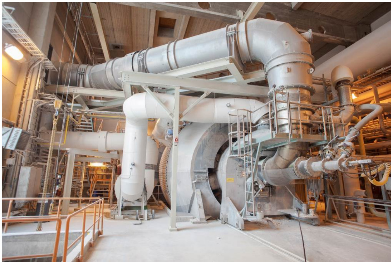
2. Multi-fuel burner used to fire gasified bark [5].
