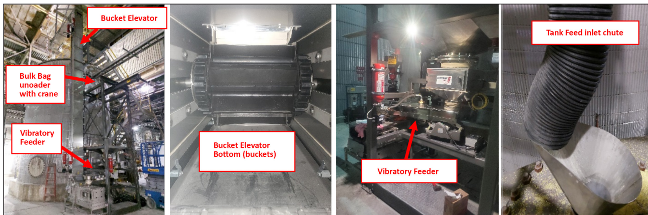
14. Sulfur addition system.
