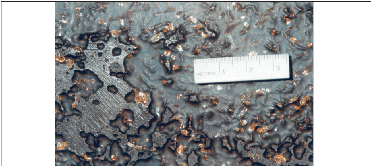
4. "Ocean-island" corrosion. Low areas drop off steeply from the high areas.
