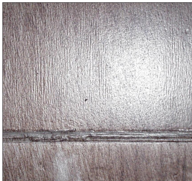
6. Grooving on the corroded surface suggests a form of erosion-corrosion. Preferential corrosion of the weld is also occurring.
