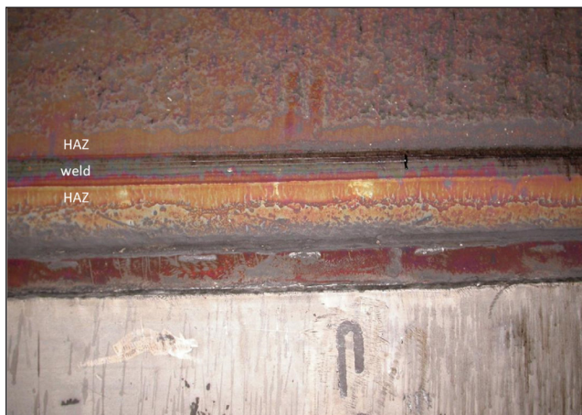
3. Preferential corrosion of a weld and heat affected zone. Rapid thinning can display a variety of colors.
